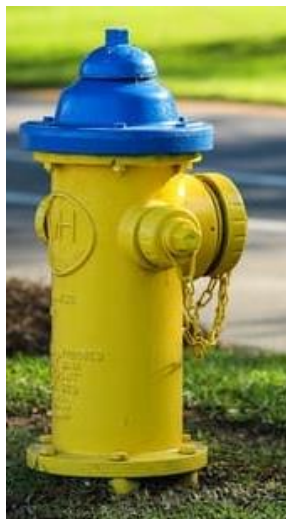
Figure 8. Example of a properly NFPA colour-coded hydrant.
